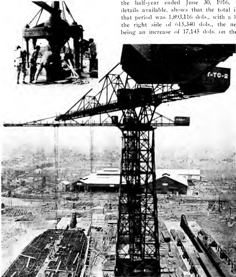
An electric bending machine is shown in the insert, while below we have a "close up" of one of the many great tower cranes with which this great yard is equipped.
